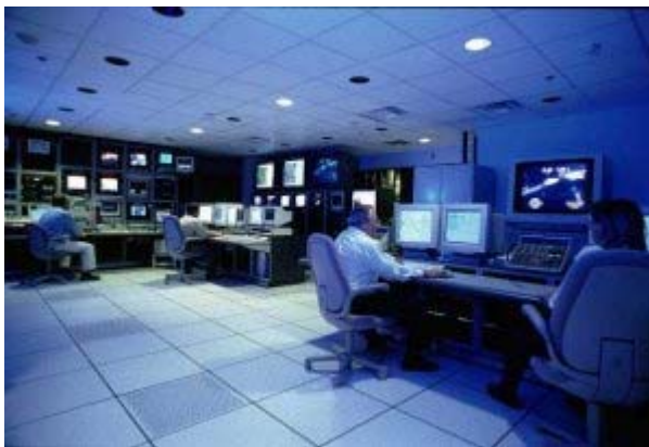
Montgomery County, MD's Transportation Management Center
